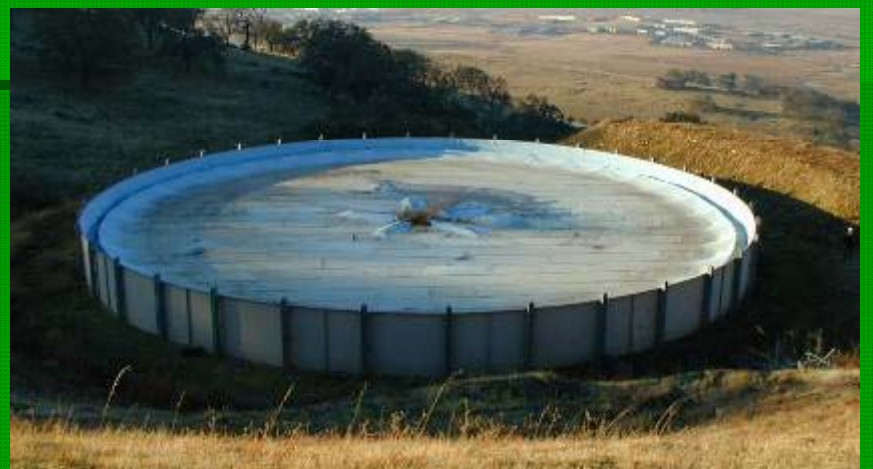
Potable water tank cover
